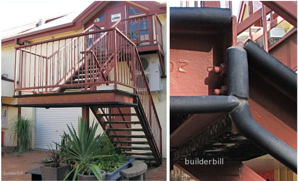
Img 11.1.1: A badly positioned half turn landing
