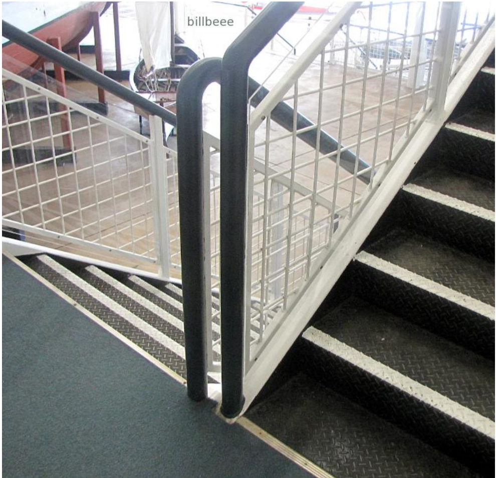
Img 8.1.8: All Steel “L” shaped
