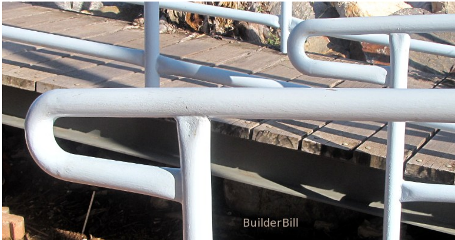
Safety terminals to rails to a ramp.
